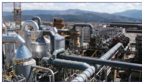
Gas cleaning plant.
